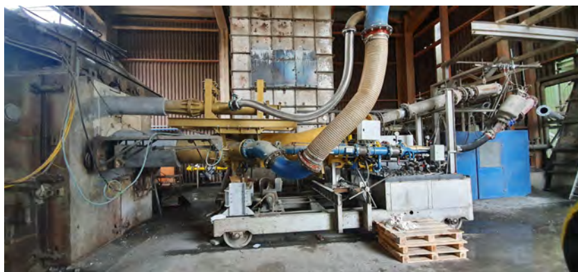
Figure 5. For the secondary fuel firing, a satellite burner DN 150 was installed.
